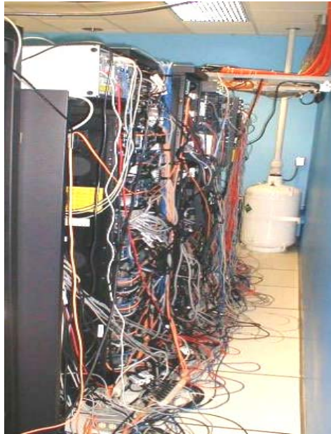
Figure 3 – Example of unstructured cabling
