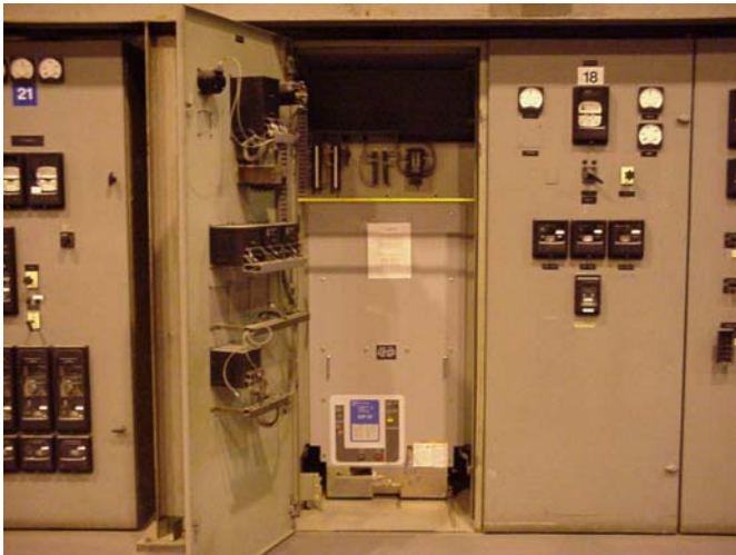
Fig. 5: Photo of the completed installation of a new replacement breaker in the upgraded "Bus A" switchgear. Original control and power wiring as well as protective relays were inspected, tested and re-commissioned.
