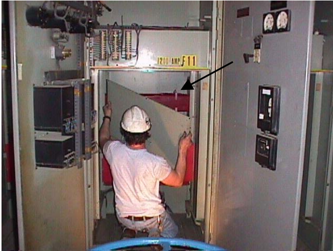
Fig. 4: A service engineer installs the main bus compartment cover plate after new bus bracing to increase interrupting rating to 1000MVA has been installed (arrow shows new bracing added in the field).
