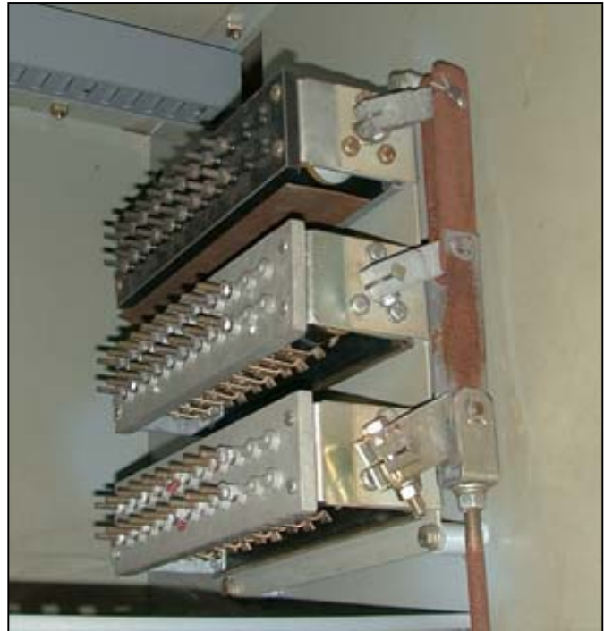
Fig. 6: Three Mechanism Operated Contacts (MOCs) mounted in a cell with mechanical (Drive Rod) linkage to the breaker operating mechanism.
