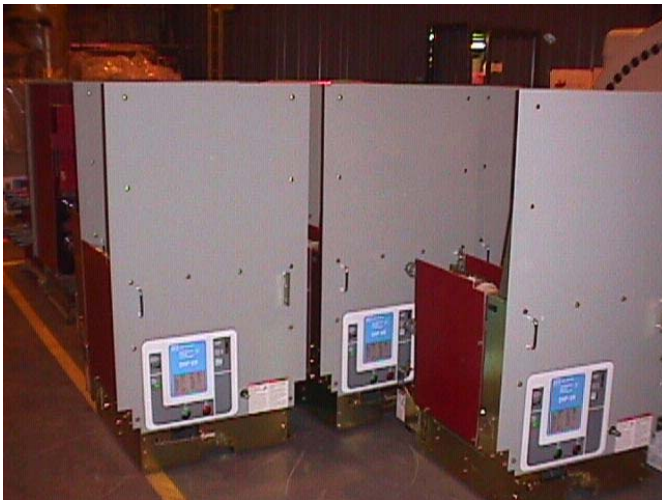
Fig. 2: Replacement breakers are positioned in staging area before scheduled upgrade.
