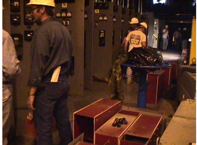
Fig. 3: During the scheduled 14 hour shutdown, a total of 2 engineers and 10 technicians from the manufacturer’s engineering services organization were deployed for the upgrade.
