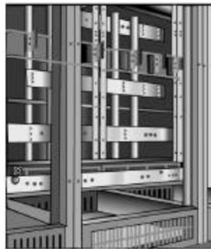
FIGURE 7: REAR VIEW OF TYPICAL LOW VOLTAGE SWITCHGEAR ASSEMBLY SHOWING A MAZE OF BUS BARS INTERCONNECTED
